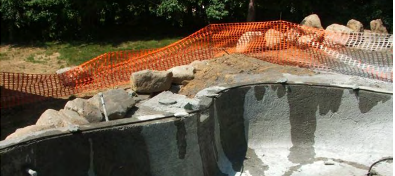
Partial wetting is not acceptable. All exposed concrete must be kept continuously wet for 7 days.
