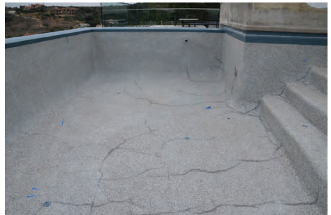
Cracking in the concrete pool shell from inadequate curing will mirror through the plaster coating.
