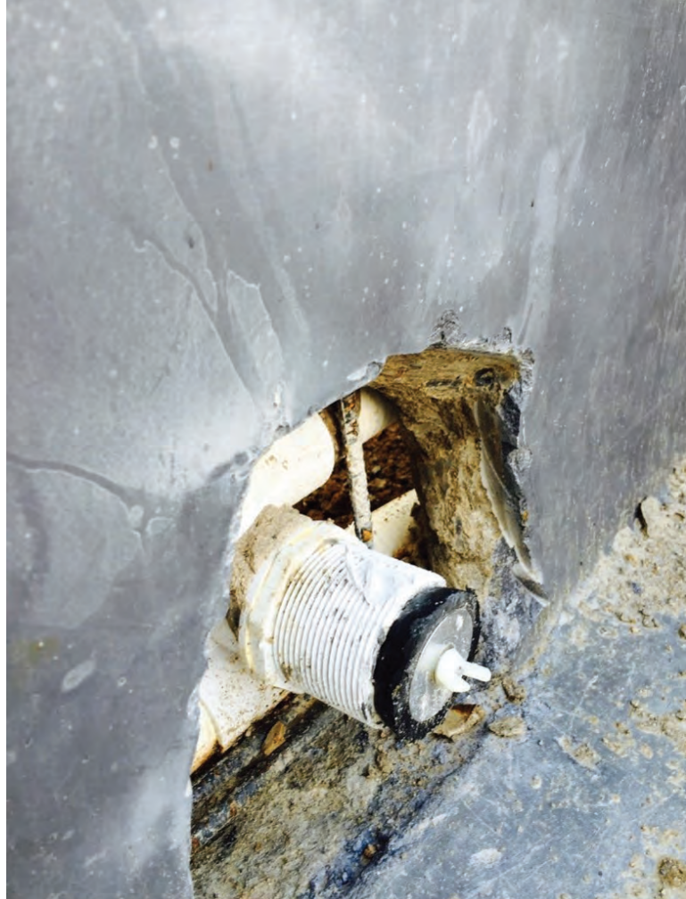
Fig. 2: Thin wall shotcrete, insufficient concrete placement and no encapsulation of surrounding penetrations or steel reinforcement
