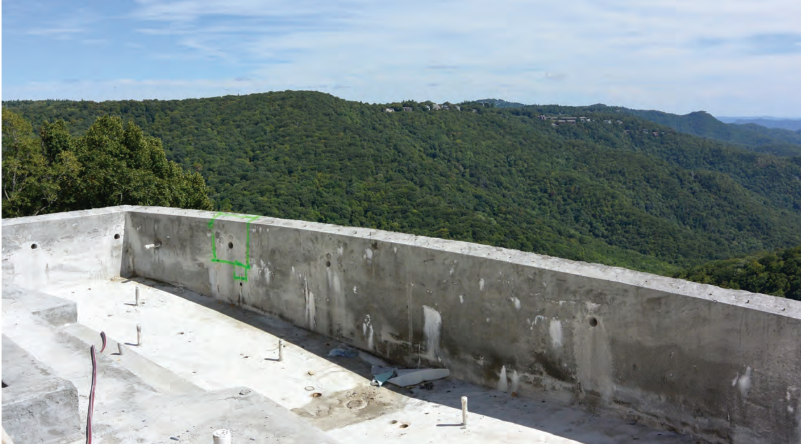
Fig. 4 Extensive efflorescence from cracks in pool shell due to design and construction issues.
