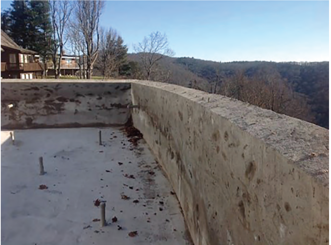
Fig. 1: Dry mix, low w/c ratio, low cementitious content, water added to floor
